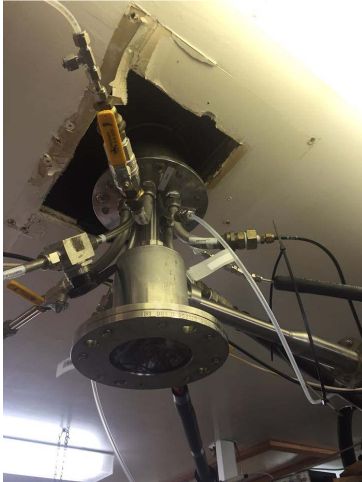
Figure 3: Aerosol splitter in the station.
